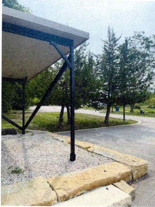
Screening at Paddleboard Structure
